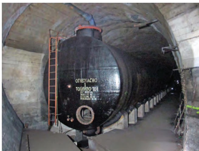
Impressive oil-storage tank still in situ at Janska Objekt H, with Cyrillic script on the butt
